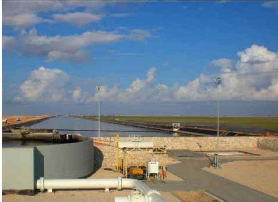
Plate 1: View from the inlet works of the Nimr water treatment system. The oil contaminated water passes through the oil separation facilities in the foreground before flowing down the long inlet buffer pond which enables even distribution of the water into the 240 hectares of wetlands, seen in the right of the photo.
