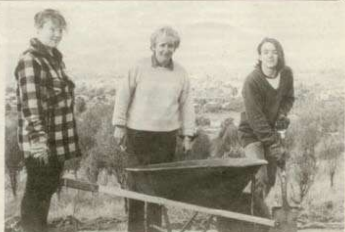
LEAP PROJECT: Young locals (left) Leonie Onn and (right) Guy Putland start work on a lookout platform on Mt Ommamey with supervision from Sandra Ryan from Greenskills.
