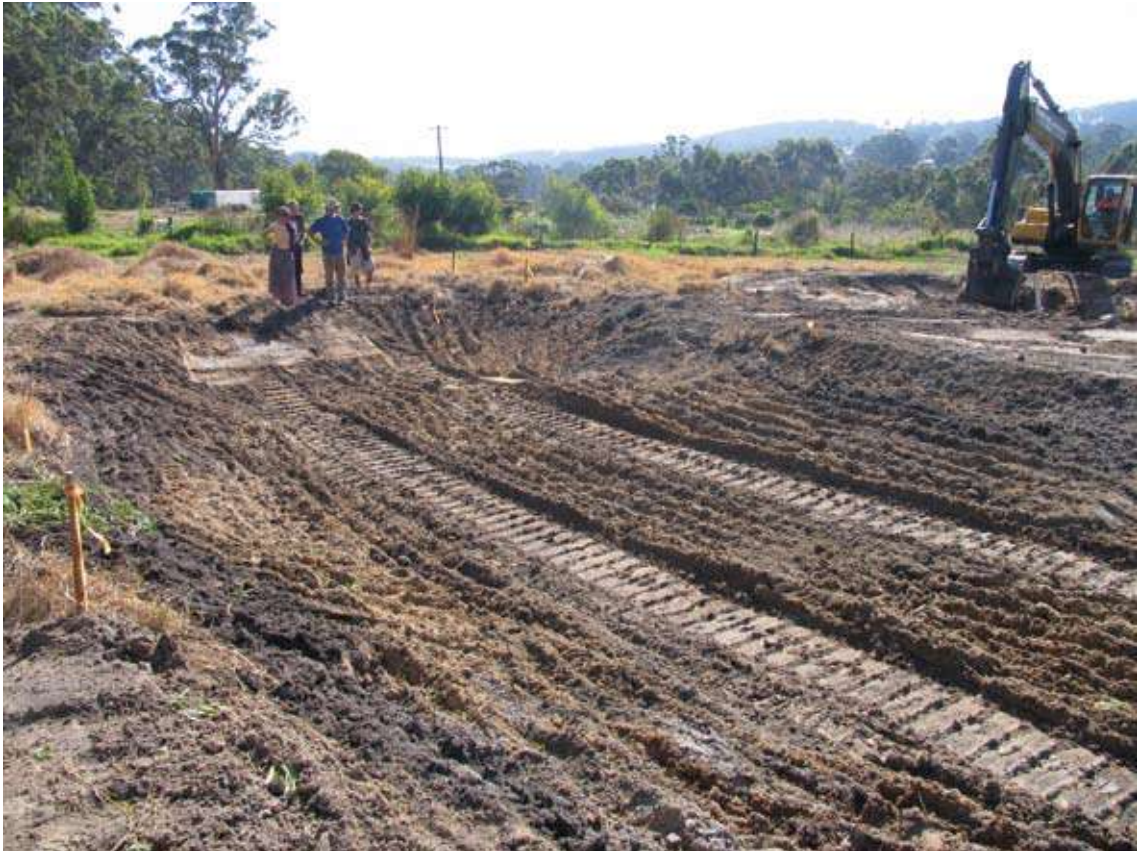
Earthworks at the site of the Centre for Sustainable Living wetland in early 2006
